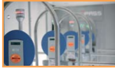
The powered SkiData turnstiles ensure comfortable and smooth operation. In case of emergency the bars collapse and provide an unobstructed exit.
