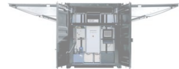
A view of the technical room in the Crowd Gate. All the control components easily accessible and securely locked behind steel doors.
