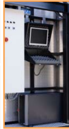
The Crowd Gate control room houses a server which can manage up to 60 turnstiles and send real-time data to other computers in the network or via the internet.
